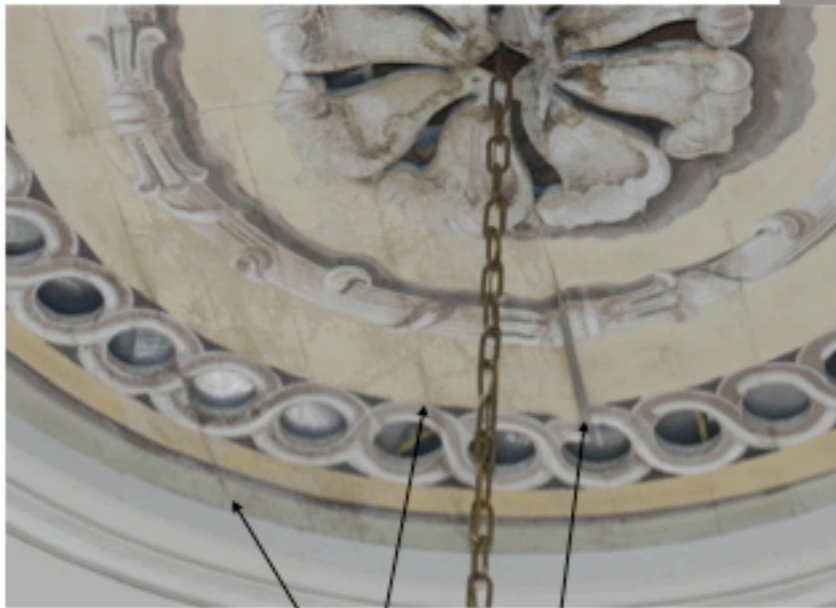
Ceiling cracked and peeling
