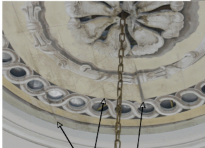
Ceiling cracked and peeling
