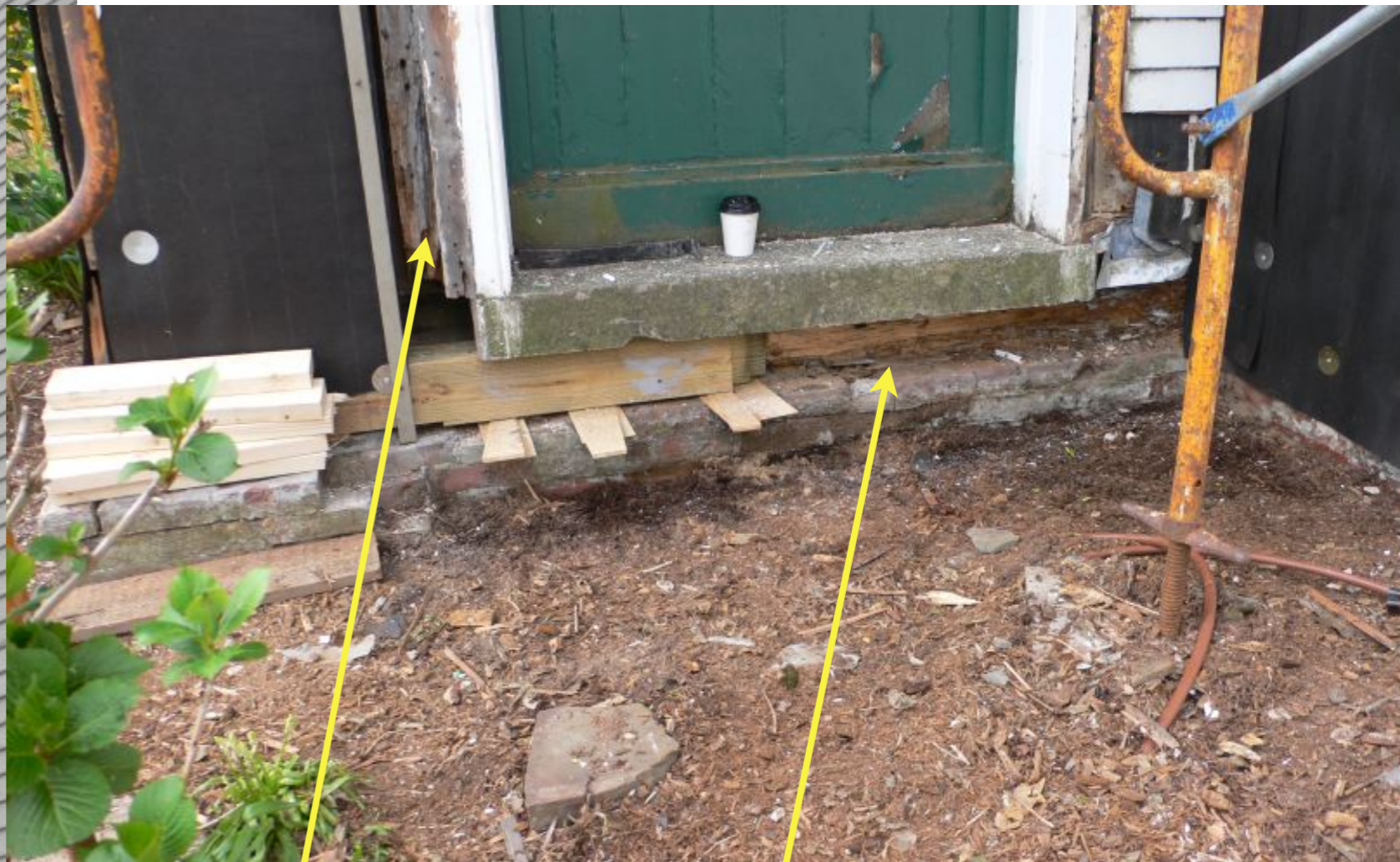
Rotted sill portion at north door of narthex, and rotted sheathing
