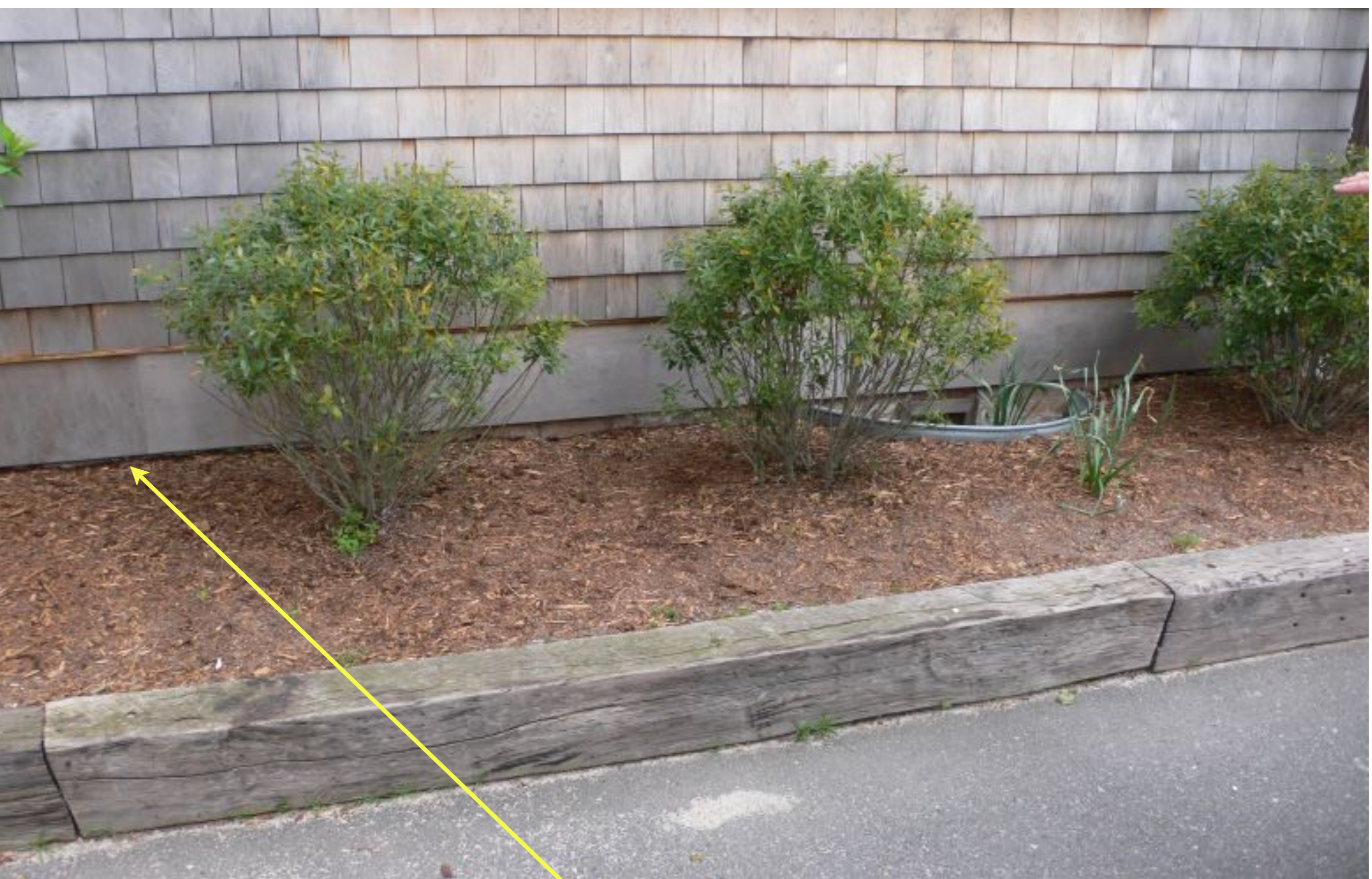
South facade at grade. Mulch piled up to wooden materials
