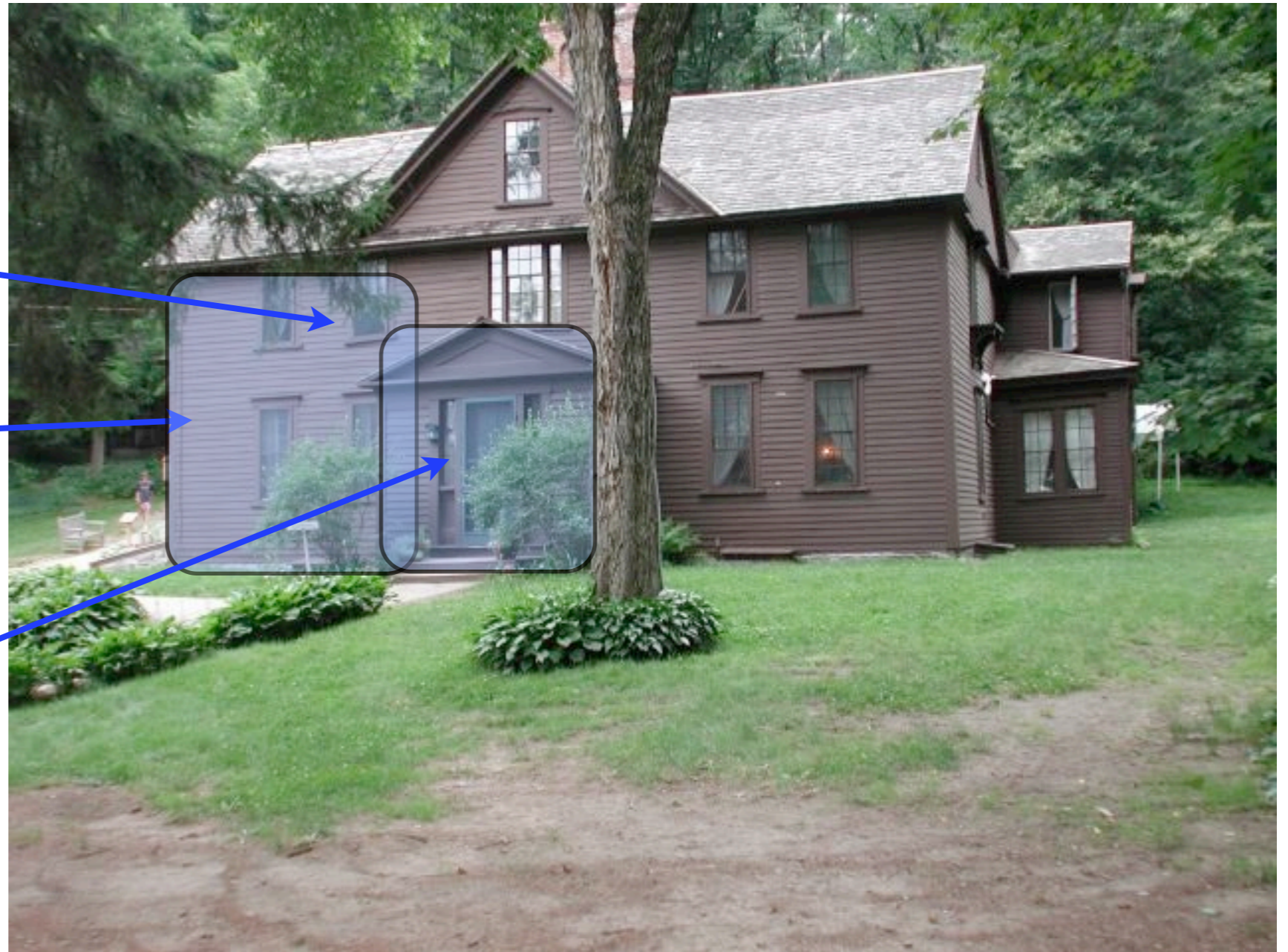
Location of needed repairs and restoration of finishes
